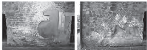
Figura 2 Reticulate façade protected using rendering at Villa Arianna (Stabiae) – outdoor face of walls
